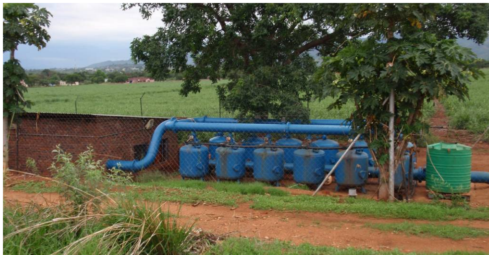
Figure 7 Primary filters for drip irrigation (Zelpy Cooperative, Buffelspruit)
