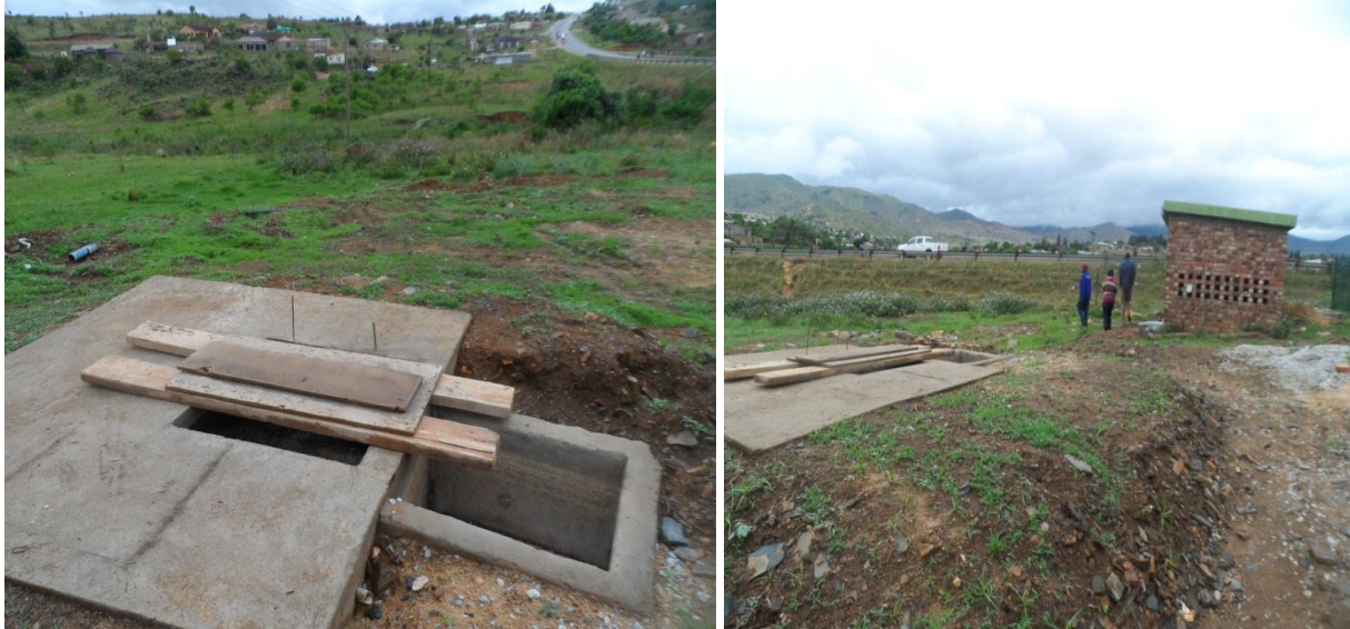
Pictures showing the septic tank during construction (left) as well as after construction
